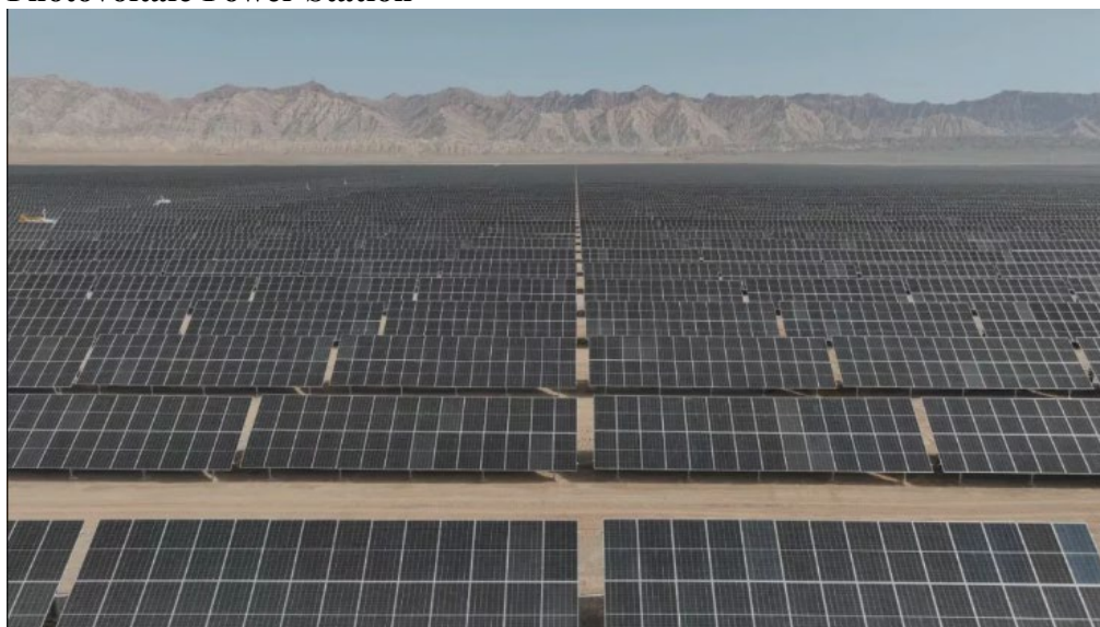
Fig. 6.3.2 Xinjiang Kuqa Green Hydrogen Demonstration Project Photovoltaic Power Station
