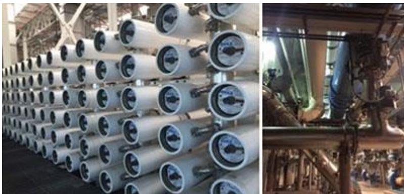
Image: Pipes, pumps and filters at the Groundwater Replenishment System. Photo by author.
