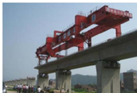
Beam Launching Equipment
