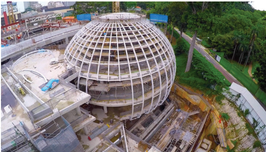
Putting the dome's structure together during construction of the Kwa Geok Choo Law Library
